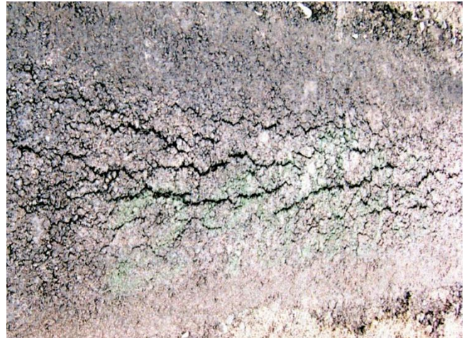
Figure 19: Cracks due to compaction of adjacent fill material (Hóeg 2009)
