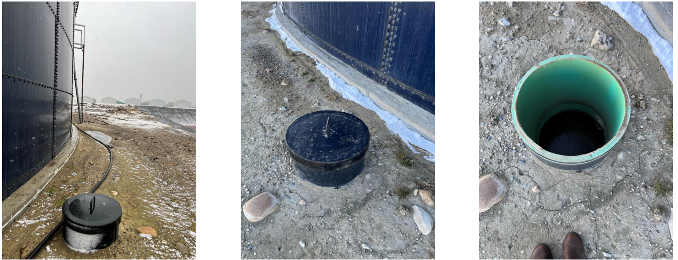
Figure 1: Three photographs depicting the slurry tank sump to be visually inspected annually, and sampled should liquid be observed.
